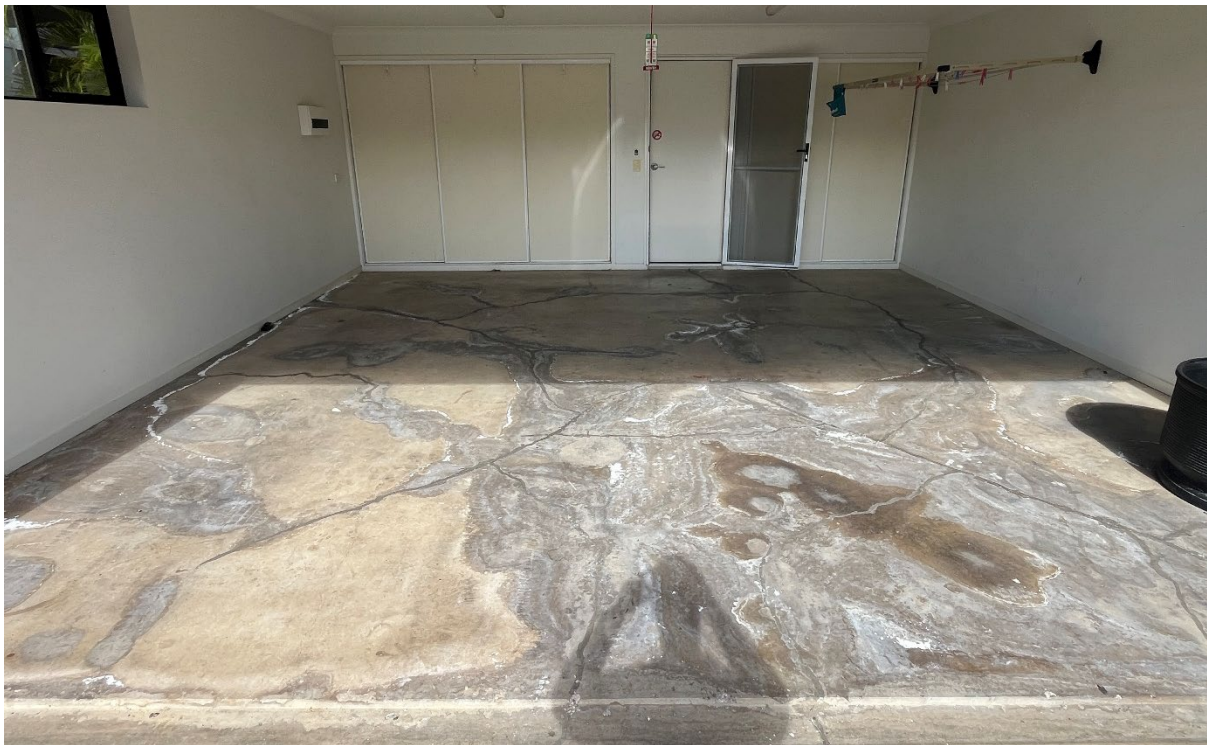
Figure 1: Figure 1 represents the context of the work area with severe efflorescence visible across the surface, and cracking suggestive of subgrade movement or degradation.
