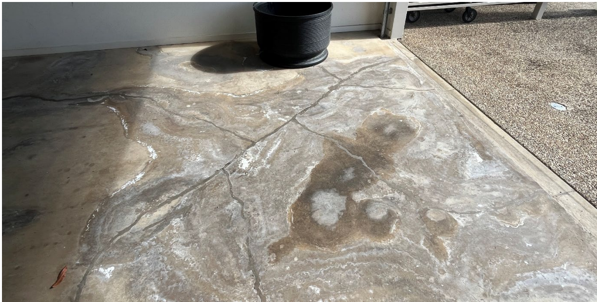
Figure 4: Figure 4 shows a localised area of surface moisture accumulation and staining, characterised by darker discolouration and associated efflorescence. The irregular shape and diffuse boundaries of the wet patch are consistent with moisture migrating through the slab rather than originating from a surface spill or isolated event.
