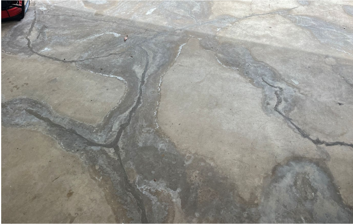
Figure 3: Figure 3 shows a close-up of the efflorescence and cracking pattern, which, due to its non-longitudinal nature, appears to indicate subgrade movement as a cause.
