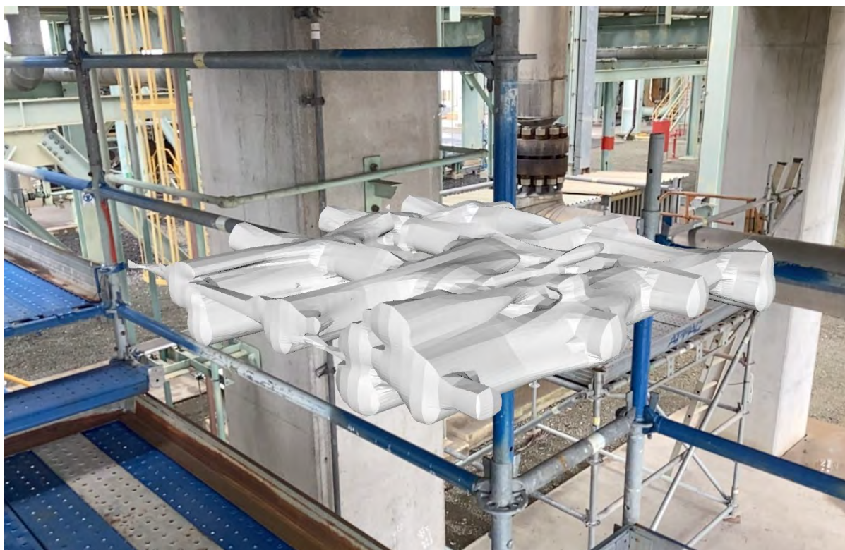
Figure 14: 3D visualisation of the slab underside, confirming the additional bar placements on the right of the image, strengthening the slab's centre in place of trimmer bars. The overlap of the multiple bars is visible.
