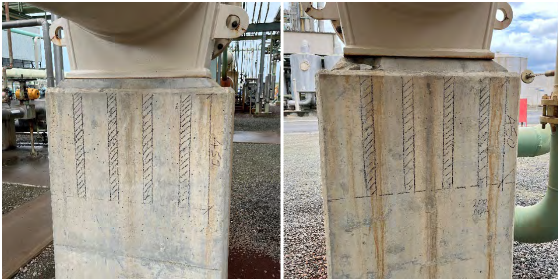
Figure 16: Bolt penetrations detected using GPR scanning on the side of the pipeline plinths. The penetrations extended to approximately 450mm, placed in the centre of the plinth with ~200mm of concrete cover.
